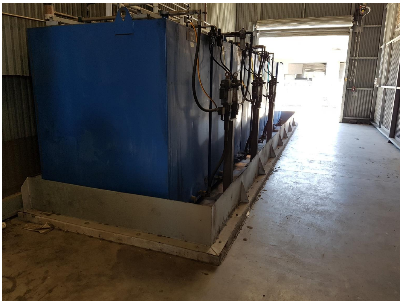
Plate 17: Engine oil bunding in Workshop
