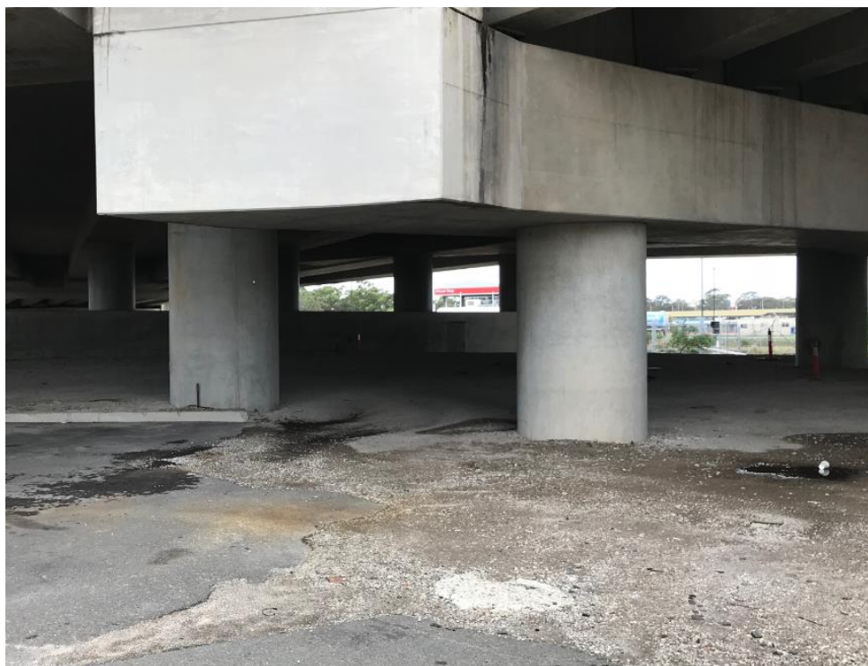
Plate 6B: Unbundled fuel drum removed from below Ramp D for disposal (After Photo)
