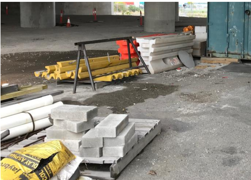
Plate 8B: Unbanded chemical containers removed from under Ramp D for disposal (After Photo)
