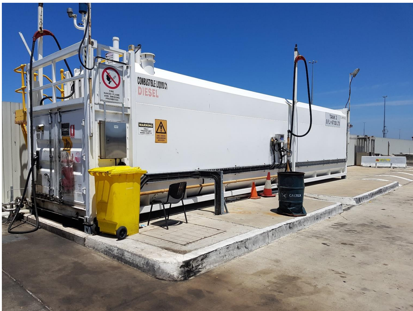
Plate 20: Double skinned bulk fuel storage tank with spill kit present
