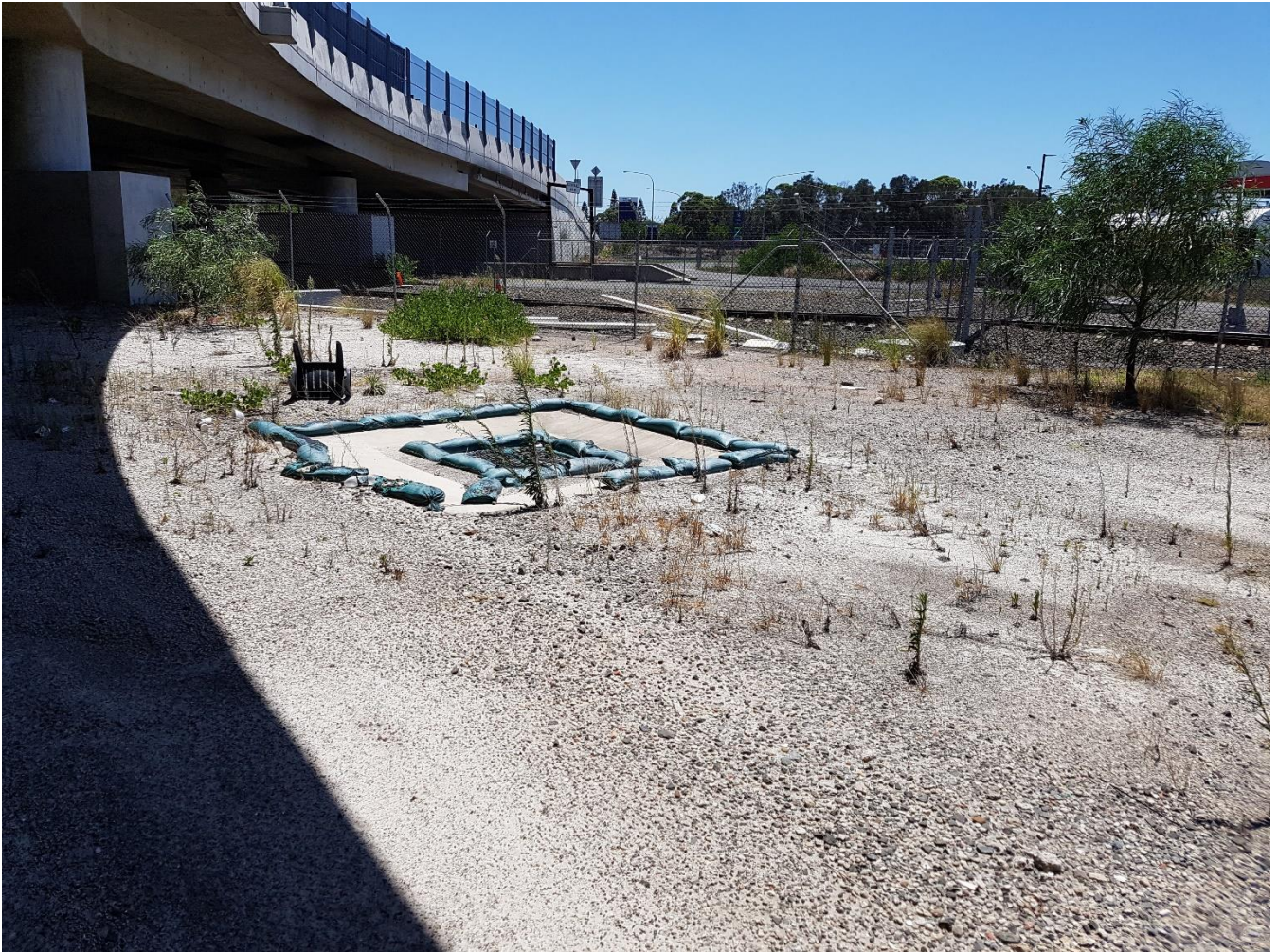
Plate 16: Landscaping in need of rejuvenation near Ramp D
