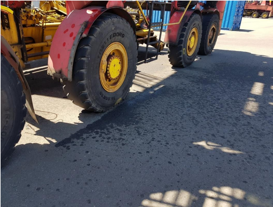
Plate 14A: Oil or fuel spillage stain from Straddle Carrier repair work at The Knuckle
