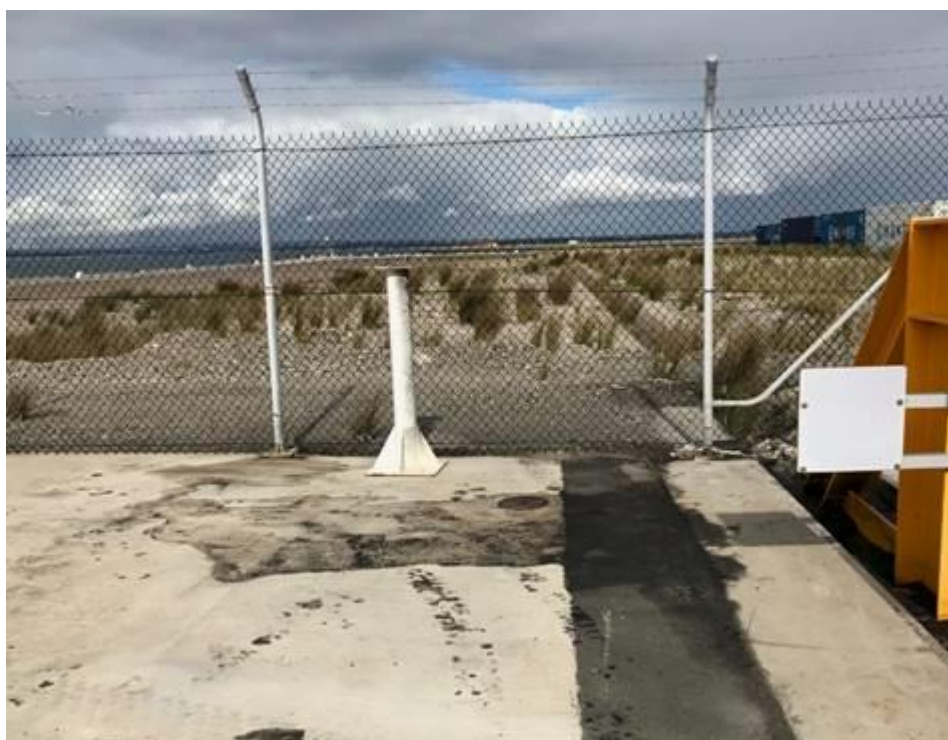
Plate 6B: Unknown residue cleaned using Hydrawash and litter removed from pavement at The Knuckle (After Photo)
