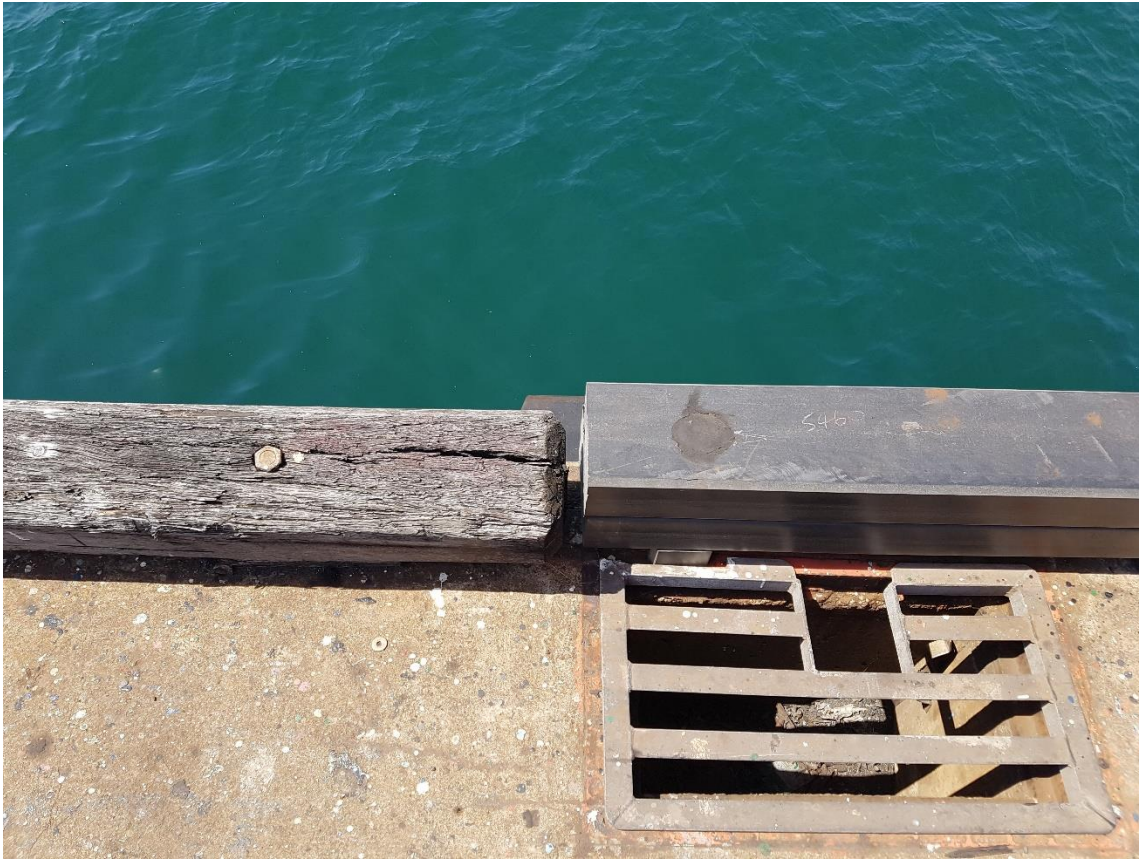
Plate 10: Recycled plastic being used to gradually replace timber stringers along the edge of the wharf
