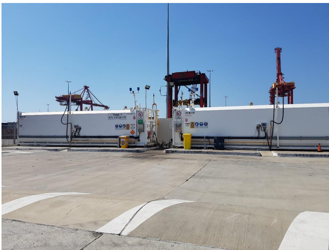
Plate 2: Double skinned bulk diesel storage tanks with spill kits near filling areas, bund (foreground) surrounds the forecourt area where diesel tankers park
