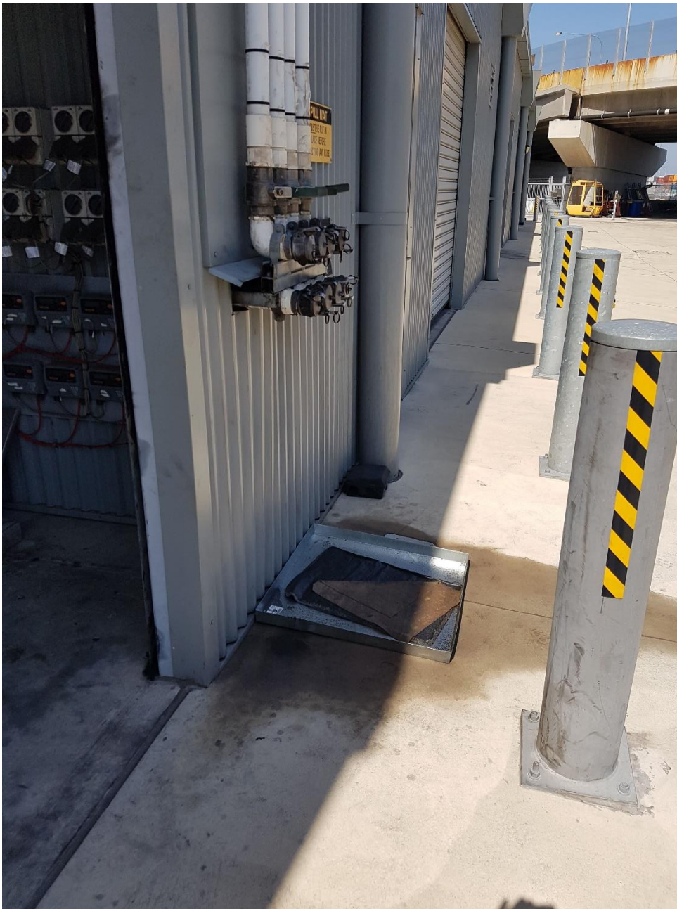
Plate 5: Drip tray under engine oil couplings at Workshop
