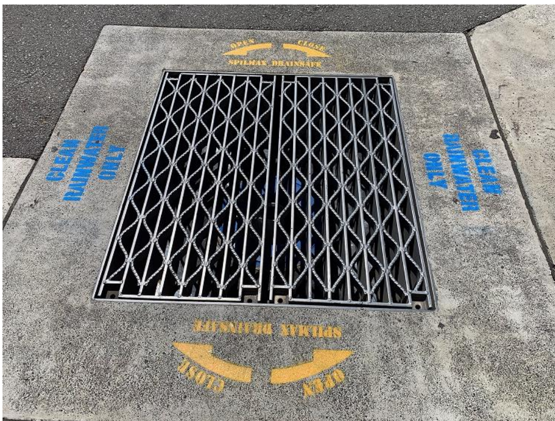
Plate 3: Drain warden device (under grate) at stormwater inlet near access road way adjacent to Gate B110
