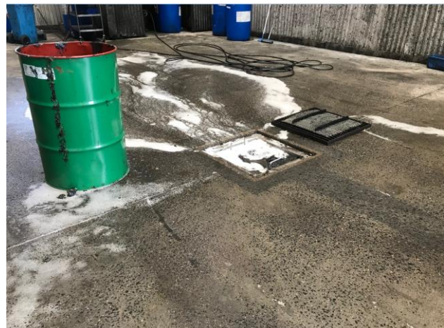
Photo 6.8.4: Wastewater from the wash bay draining into a sump which drains to the wastewater holding tank.
