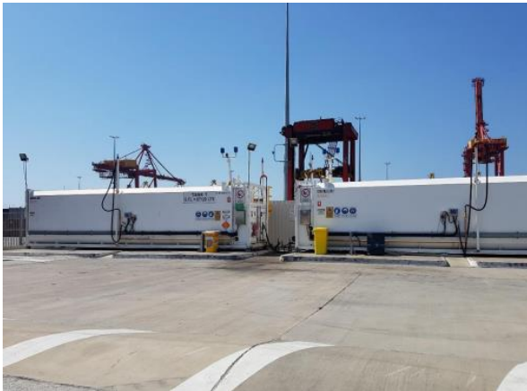
Photo 6.6.1: Diesel trans-tanks in bunded area
