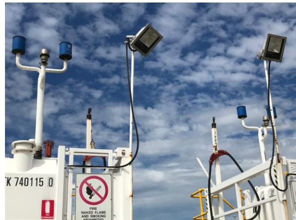
Photo 6.5.2: Diesel storage tanks – relief valves and filters
