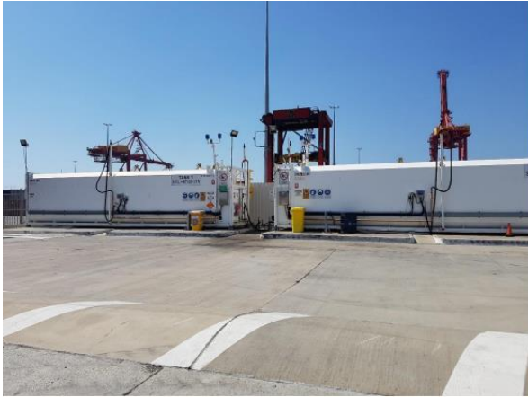
Photo 6.5.1: Diesel storage tanks
