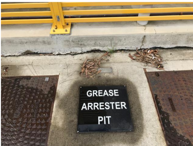
Photo 6.8.3: Grease Arrester Pit (Permit No. 40110) collects greasy wastewater from the Canteen/Kitchen.
