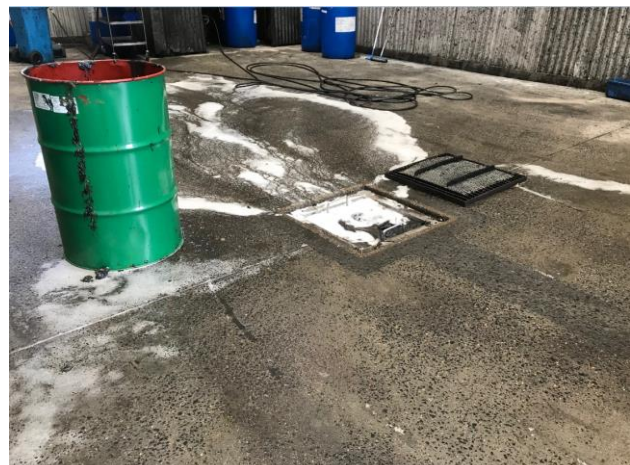
Photo 6.8.4: Wastewater from the wash bay draining into a sump which drains to the wastewater holding tank.
