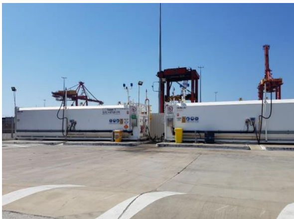
Photo 6.6.1: Diesel trans-tanks in bunded area
