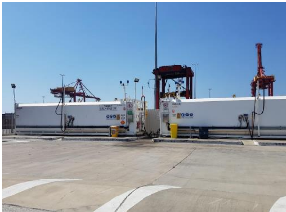
Photo 6.6.1: Diesel trans-tanks in bunded area
