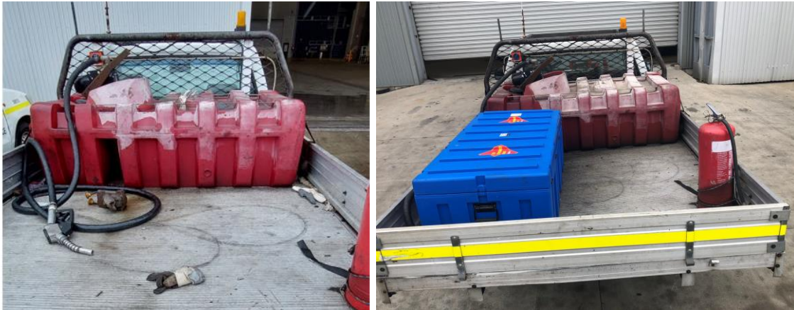
Site Photo 9A and 9B Mobile refuelling tank on Maintenance light vehicle, with no secondary containment or spill kit, and the action taken by Patrick to install a spill kit on this vehicle (prior to finalising this Audit Report). Note Site Photo 9B provided by Patrick.
